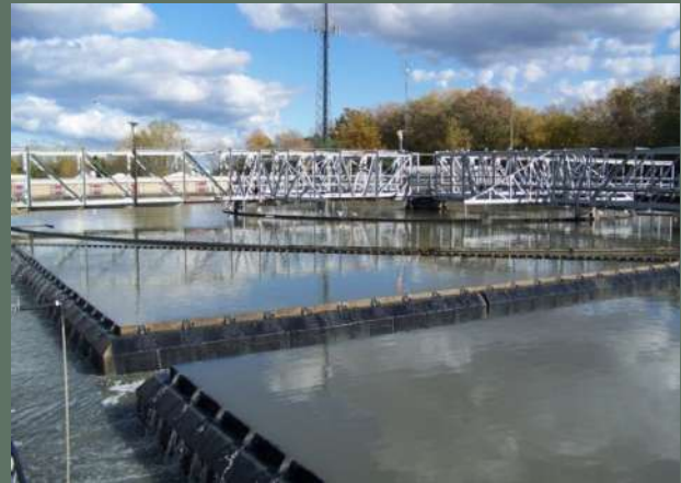
Monroe County Water Resource Recovery Facility
