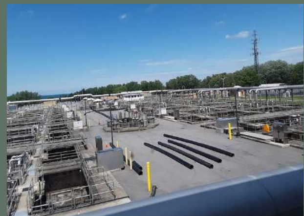
Monroe County Water Resource Recovery Facility
