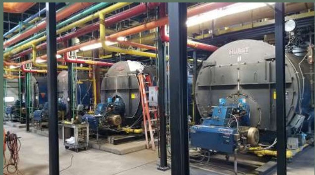
Iola Powerhouse & Cogeneration Facility
